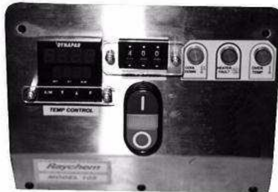
Front of Control Enclosure
